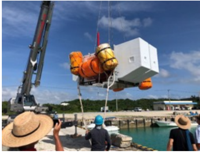
Figure 1. Taper-Ducted OIST - Wave Energy Converter Device surrounded by floaters being lifted into the water using crane to be towed to the installation location using a boat.
