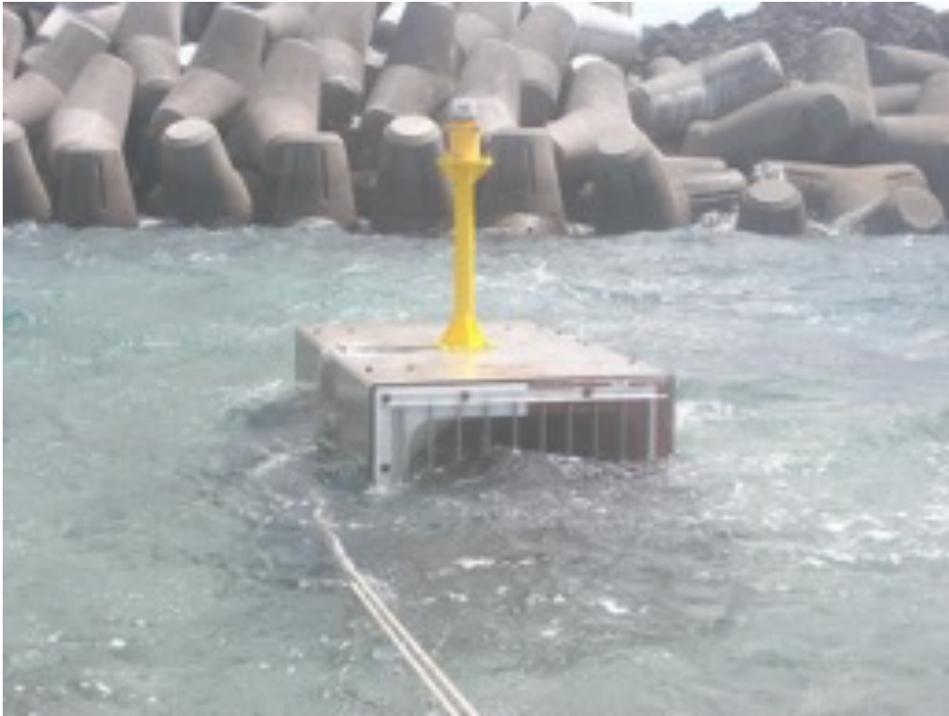
Figure 25 The complete structure after installation at the Port of Seragaki. A small LED beacon is fixed on the top of the structure to warn passing ship or boat of the structure's existence especially during the night.
