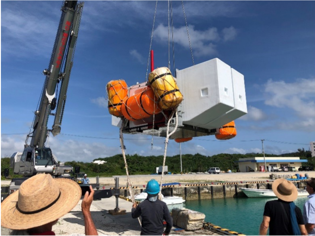
Figure 24 The complete structure of the WEC surrounded by floaters being lifted into the water using a heavy machinery. The complete structure is light enough to be towed the designed location using small boat.
